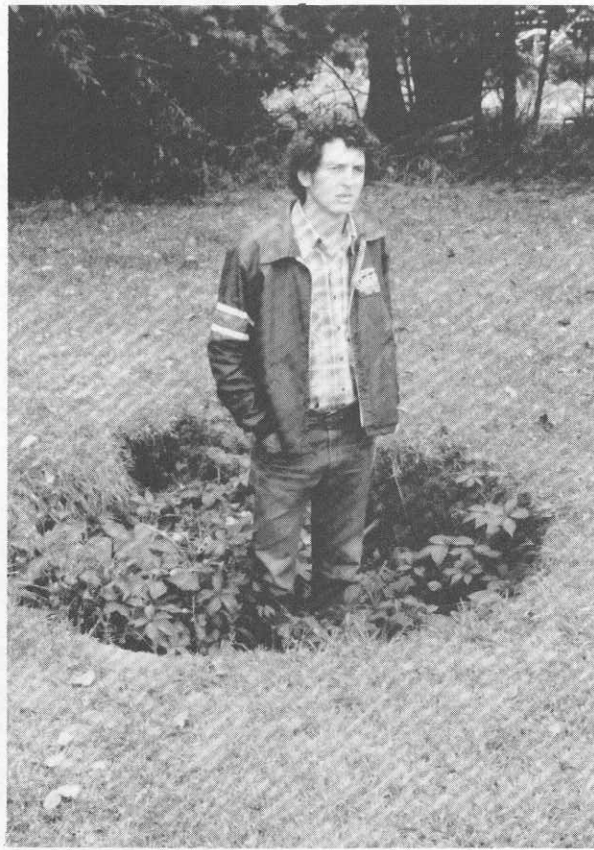
Photo No. 9 Crater above What Cheer Coal Co. F., SW, NE, SW, Sec. 10, T76N, R13W. View is roughly southeast.
