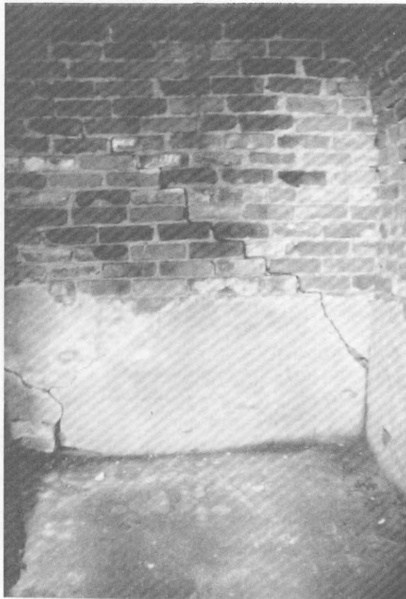
Photo No. 13 Interior of root cellar, north wall, above What Cheer Coal Co. F., NE, NW, SW, Sec. 10, T76N, R13W. View is north.
