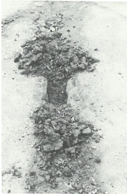
Figure 6. Till-packed joint in the limestone. Joint is about 5 inches wide.
