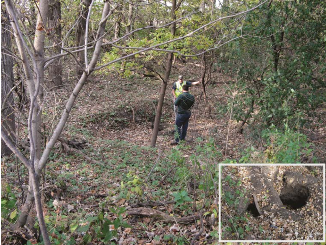
Fig. 3: A developing sinkhole found in the mapping area. The lower-right picture shows the central hole of the structure.
