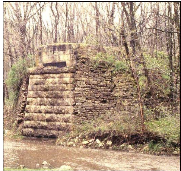
Figure 1. Old railroad bridge pier along Otter Creek west of the picnic area.
