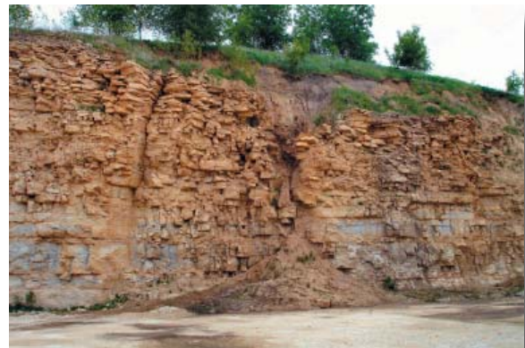
Figure 3-3. Skyline Quarry. Note sinkhole in cross section.
