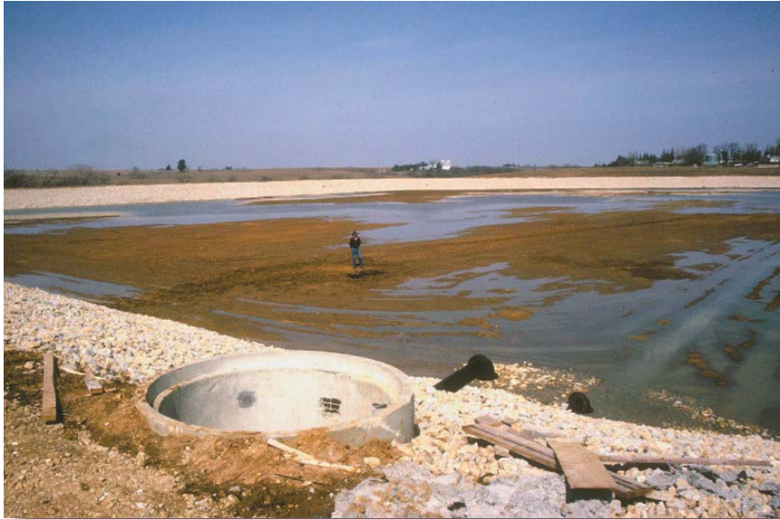
Figure 1-2. City of Garnavillo lagoon after sinkhole failure.
