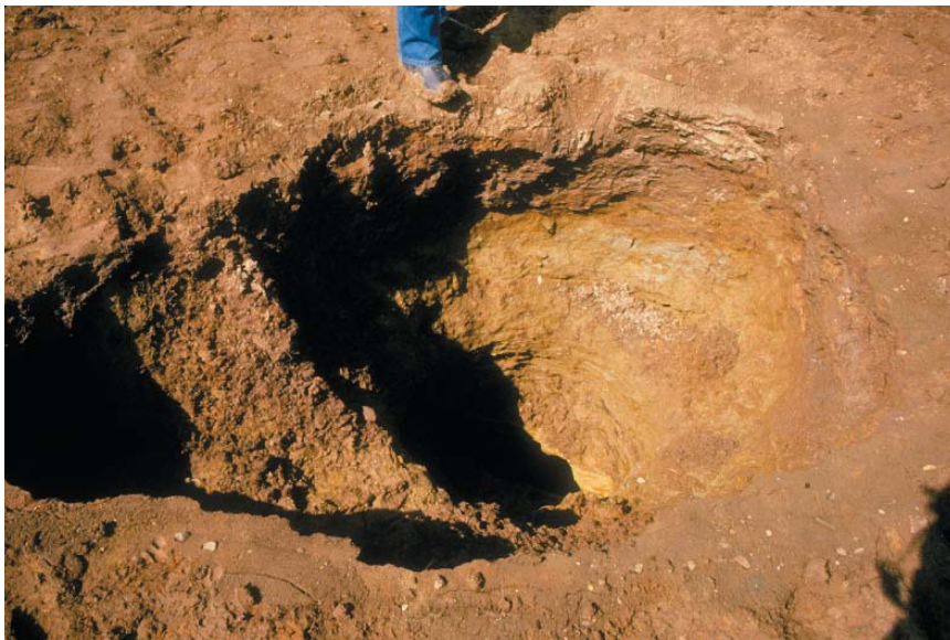
Figure 1-3. Close-up of sinkhole at City of Garnavillo lagoon.
