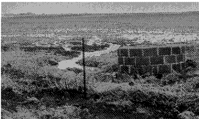
Figure 3. An ADW in Humboldt County, Iowa. The top of the cistern is in poor repair and has no cover. (Photo courtesy of the Iowa Environmental Council.)
