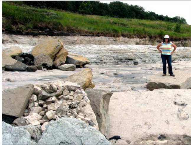
Figure 6. Coarse limestone aggregate used in the post-1993 spillway reinforcement can be seen in the overturned concrete slab on the left. For scale DOT geologist Adriana Reyes-Phelps stands on the right.
