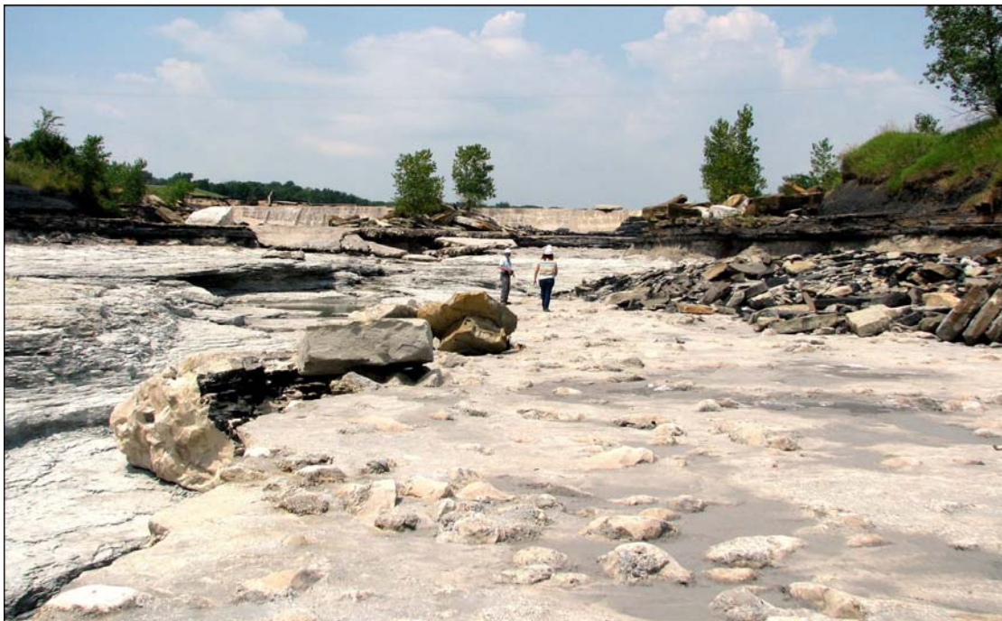
Figure 7. View of the Upper Gorge of the Saylorville emergency spillway as exposed after the 2008 floods. Stop 2 of the field trip will be in this area. The material in the lower right is concrete installed to stabilize the spillway after the 1993 floods. The structure in the background is concrete lip of the spillway.
