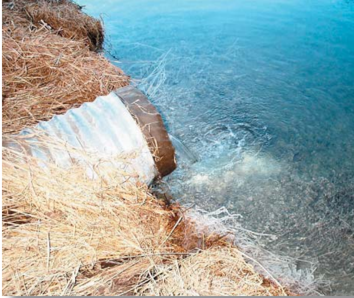
Contaminants often travel through tile lines into streams, resulting in fish kills.
